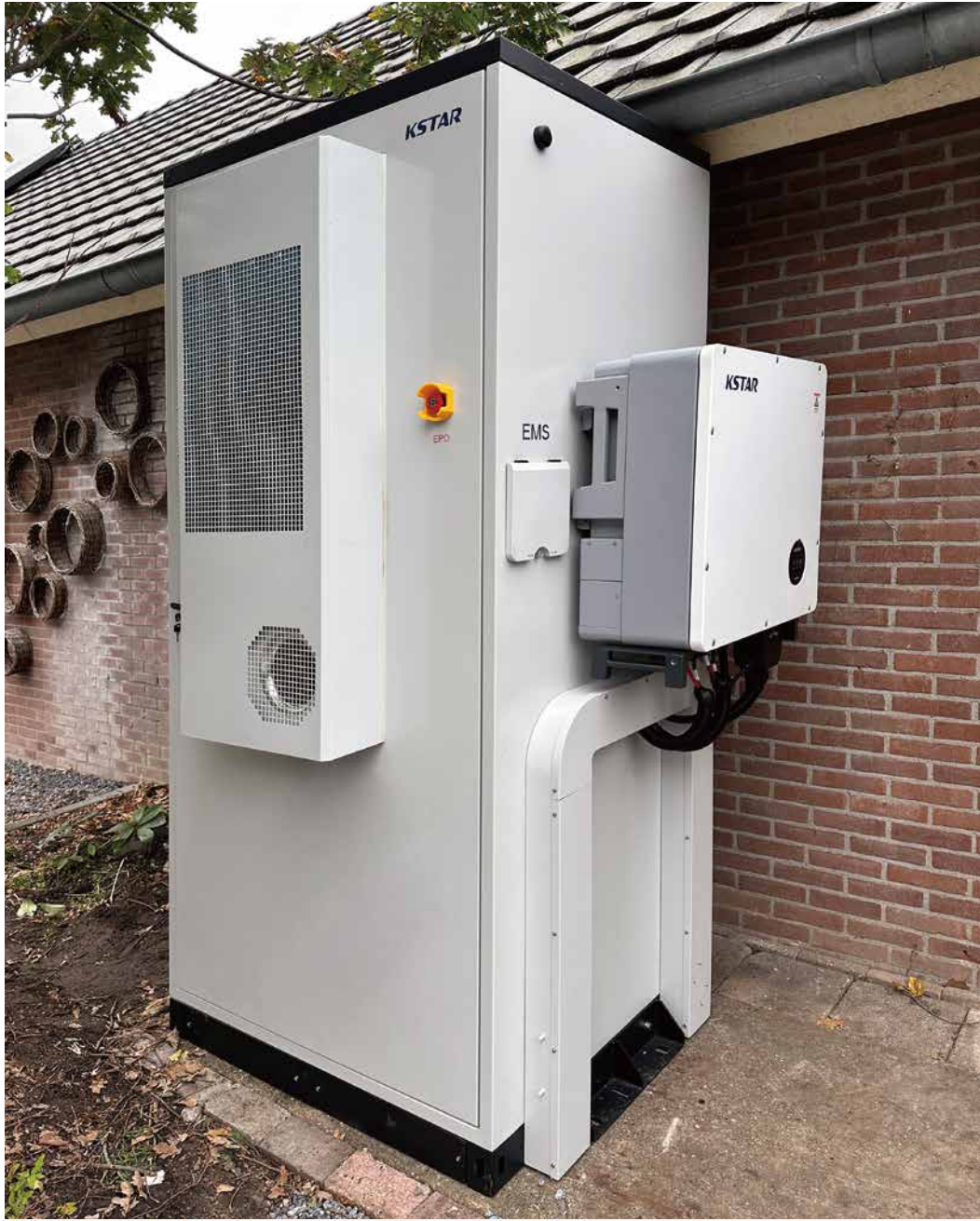
03 C&I ESS Project in the Netherlands
