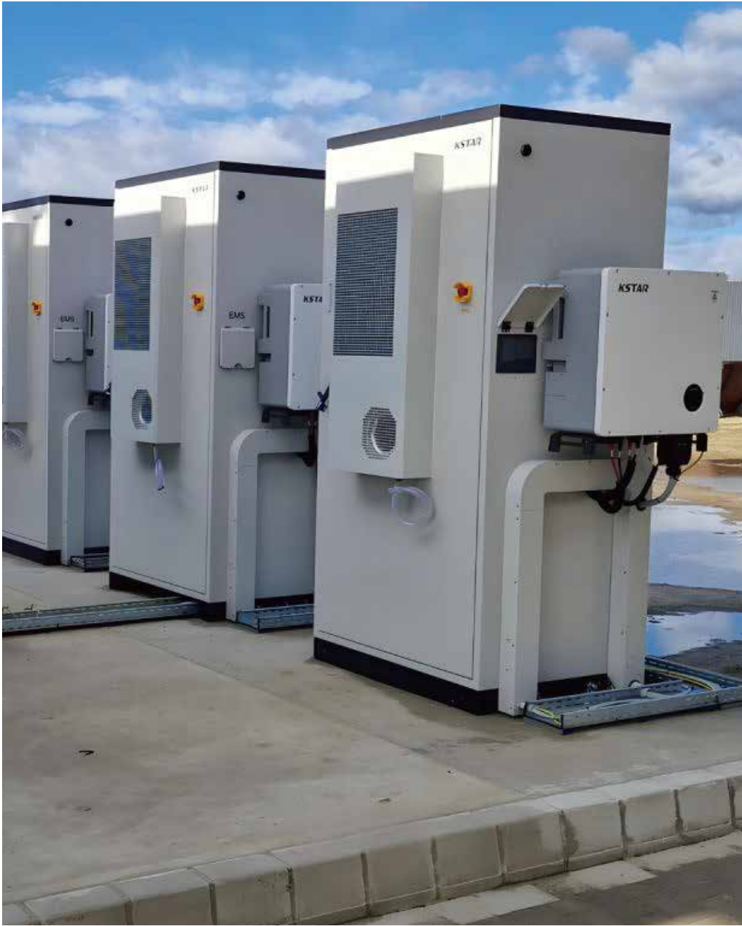
02 C&I ESS Project in Hungary
